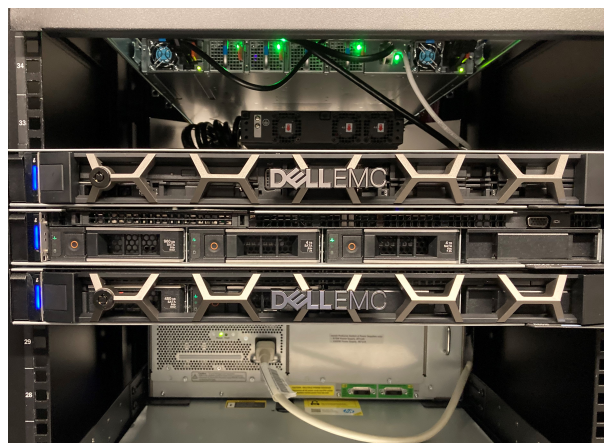
Fig. 3: A prototype rack implementation (rear view). From top: a 48 and 12 port 10/100G ethernet switch NPB access fabric; 3 1U servers functioning as a) an appliance performing payload obfuscation, b) a software packet mangler and traffic manager, and c) an NPB controller and traffic generator; and a control network switch.
